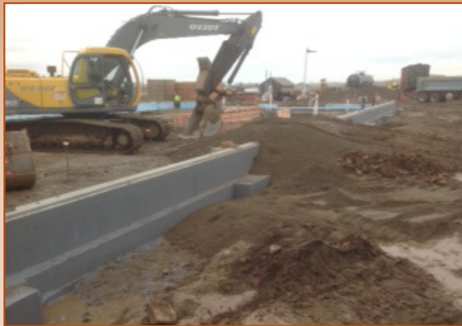
MJM Grand building a ramp over the stem wall to grade slab
